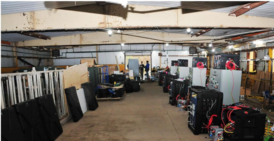
Figure 2. RADICS Substations-In-A-Box crankpath being restored as part of the exercise at Plum Island, NY in October 2020
