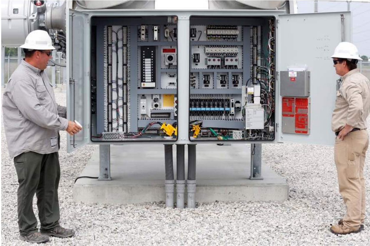
Figure 25: Substation Circuit Breaker Cabinet. Cables exit the underside of the circuit breaker control cabinet, passing underground to relays located in a substation control house. Even buried cables would conduct the E1 pulse into the cabinet and into the relays. Photo credit: The Toledo Blade.
