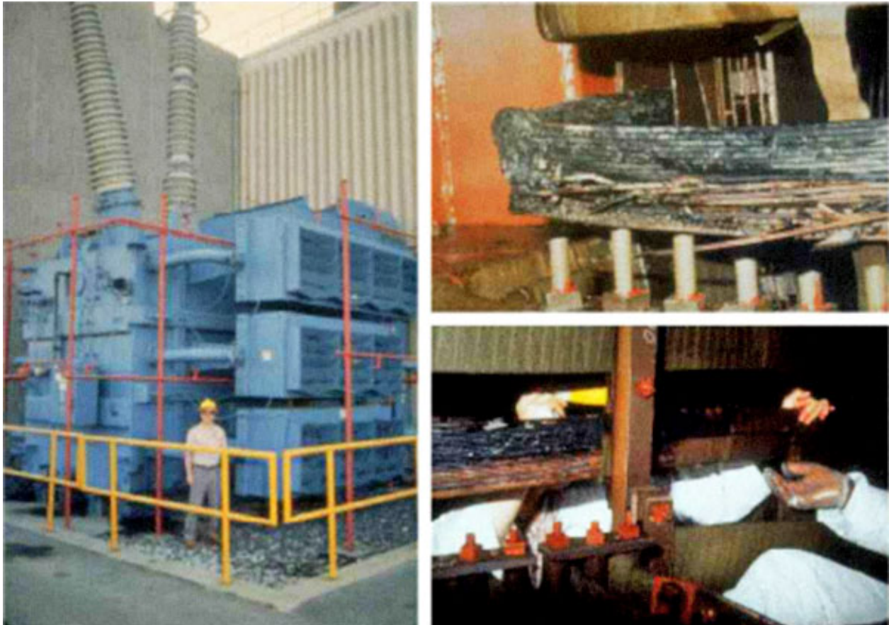
Figure 23: Failure of Salem Nuclear Plant GSU Transformer. Pictured below is one of the three single-phase transformers at the Salem Unit 1 nuclear plant. This transformer failed shortly after the March 13, 1989 solar storm. Geomagnetically-induced currents in transmission lines conducted into the transformer windings, causing saturation and overheating. Forensic examination showed charred insulation and melted windings. Photo credit: PSE&G.
