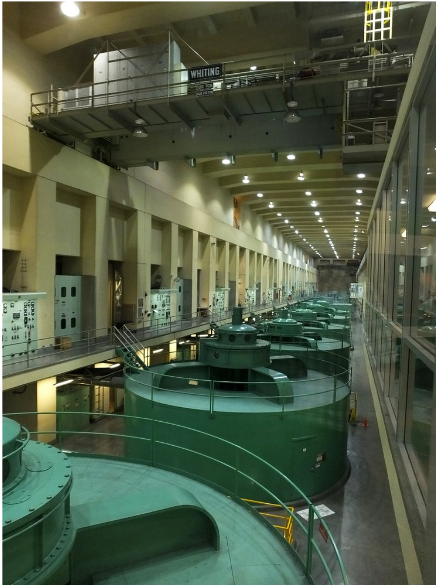
Figure 10: Generator Hall at Grand Coulee Hydroelectric Dam. This photo of the Grand Coulee generator hall shows the original analog control panels to the left of the row of generators. Analog controls can still be used to run this plant. Instructions are communicated to manual operators by means of telephones on the control panels. This extremely simple system may continue to function following a HEMP attack. Photo credit: Creative Commons/Linda Moving Ahead .
