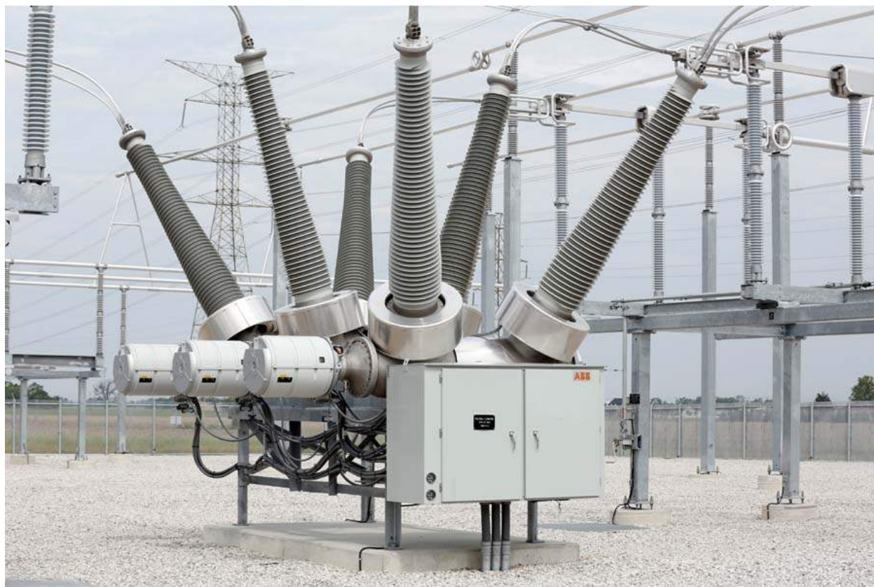
Figure 24: Substation Circuit Breaker. This gas-insulated circuit breaker interrupts all three phases of high voltage electricity. Note the exposed control cables underneath the breakers that would conduct the E1 pulse into the gray-colored circuitry cabinet. Photo credit: The Toledo Blade.
