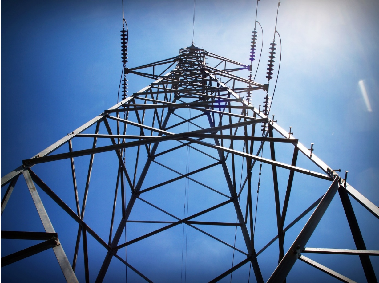
Figure 17: Transmission Tower, Insulators, and Lines. A common method of constructing high-voltage transmission lines is to use steel towers that support aluminum conductors. Ceramic insulators isolate the conductors from the towers. During the E1 pulse, an electrical arc may be established over the ceramic insulators to electrical ground, persisting after the pulse ends and causing catastrophic insulator failure. Vulnerability of modern insulators needs engineering study. Photo credit: Pixabay .
