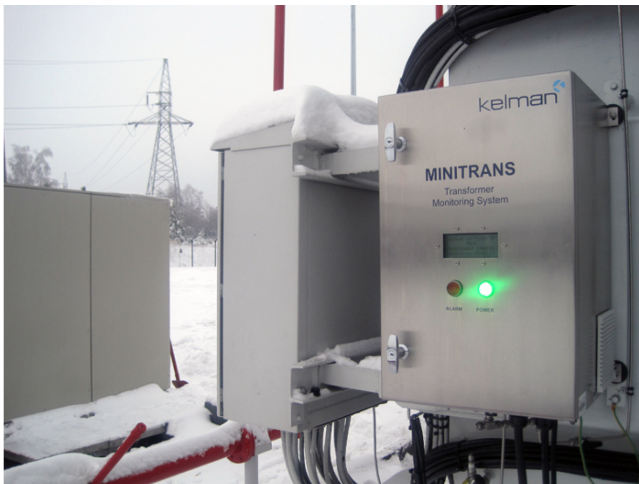
Figure 22: Transformer Monitoring System. Transformer monitoring systems collect and analyze data, presenting alarms when abnormal conditions are detected. While data from these monitoring systems would be extremely useful during a HEMP or GMD event, the copper wiring used for sensor cables can conduct the E1 pulse into monitoring system cabinets. Photo credit: GE Digital Energy
