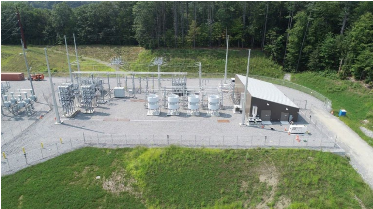
Figure 29: Static VAR Compensator Capacitor banks are on the left of the facility reactors in center. The building on the right contains controls for switching capacitors and reactors to provide lagging or leading power factor. The digital controls for SVCs are likely to be vulnerable to the E1 pulse. Photo Credit: T&D World.
