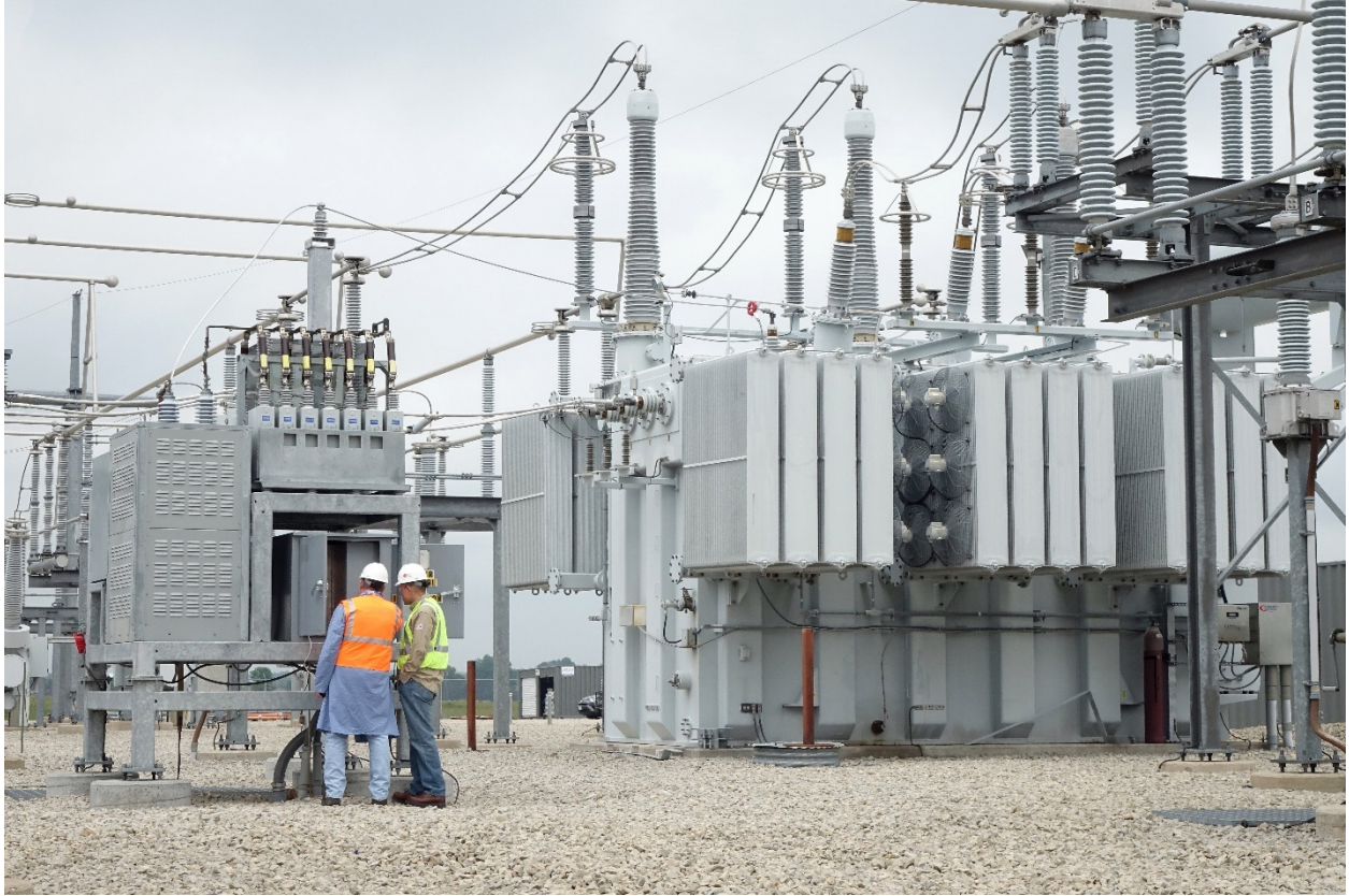
Figure 37: Neutral Ground Blocking Device. Utility workers examine a neutral ground blocking device installed to left of step-down transformer in an operational transmission system. This device blocks harmful GIC and prevents transformer oversaturation, overheating, and harmonic production. Installation of these devices at key grid nodes could protect against both E3 and GMD. Photo credit: Emprimus
