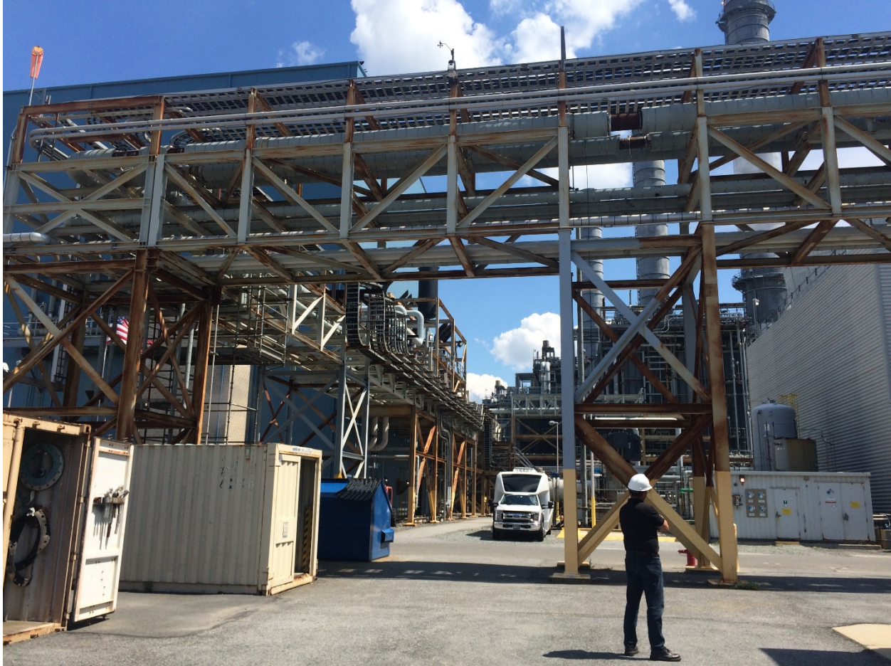
Figure 16: Control System Cabling for Combined Cycle Power Plant. Combined cycle power plants often have open-air designs with exposed control system cables running in open troughs between plant components and buildings. Note the exposed cable troughs at the center of this photo taken at a gas-fired generation plant. Photo credit: Foundation for Resilient Societies
