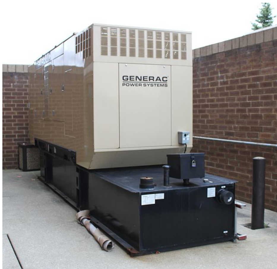
Figure 35: Backup Diesel Generator. Backup diesel generators can provide emergency substation power for circuit breakers, relays, and other control equipment. However, without specific design for EMP protection, generators can be vulnerable to the E1 pulse. Note the ventilation grates on the front and side of this metal enclosure that prevent the enclosure from providing Faraday cage shielding. Photo Credit: Wikimedia Commons/Dwight Burdette .
