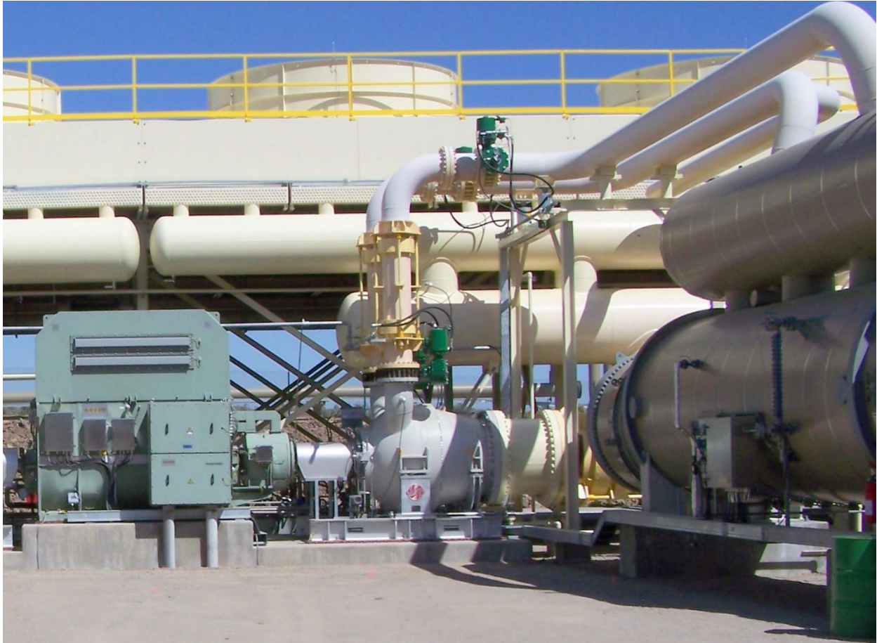
Figure 12: Control Equipment at Geothermal Plant. This photo shows pipes and control equipment at the Steamboat Springs geothermal generation plant south of Reno, Nevada. Note the exposed sensor and actuator wiring that may conduct the E1 pulse into the green control cabinet. Buried wiring ducts exiting the control cabinet (bottom left) may also expose plant-level communications to the E1 pulse. Photo credit: Creative Commons/Rjglewis
