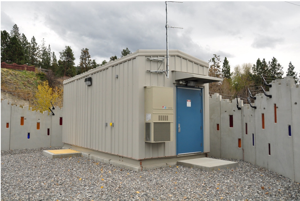
Figure 30: Exterior of Substation Control House. Sheet metal is often used to construct substation control houses. Note the HVAC unit hung on the exterior wall of the control house; these units can have digital circuitry vulnerable to the E1 pulse. Photo credit: Creative Commons/Paul Chernikhowsky .
