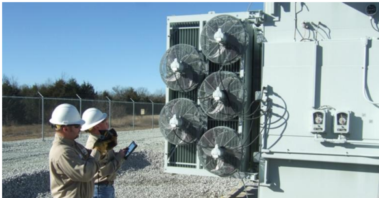
Figure 21: Cooling Components for Power Transformer. Power transformers commonly have oil pumps, radiators, and cooling fans. The exposed electrical wiring for these fans will conduct the E1 pulse into control circuitry for the transformer. Photo Credit: T&D World
