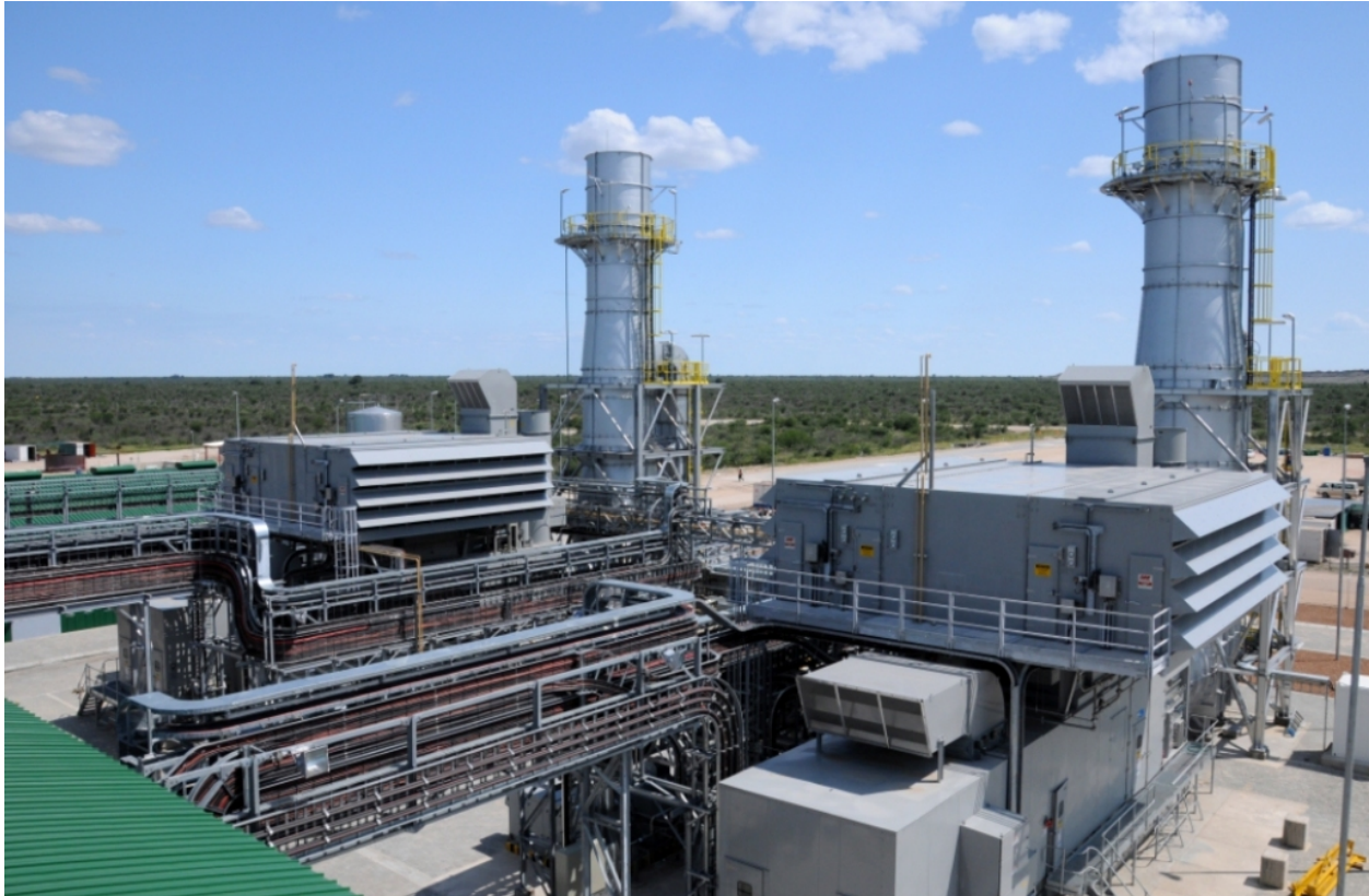
Figure 6: Natural Gas-Fired Generation Plant. Photo shows a natural gas-fired generation plant with modular design. Use of open cable troughs (center) leaves control systems potentially vulnerable to the E1 pulse. Photo credit: Wikimedia Commons/Pro-Per Energy Services
