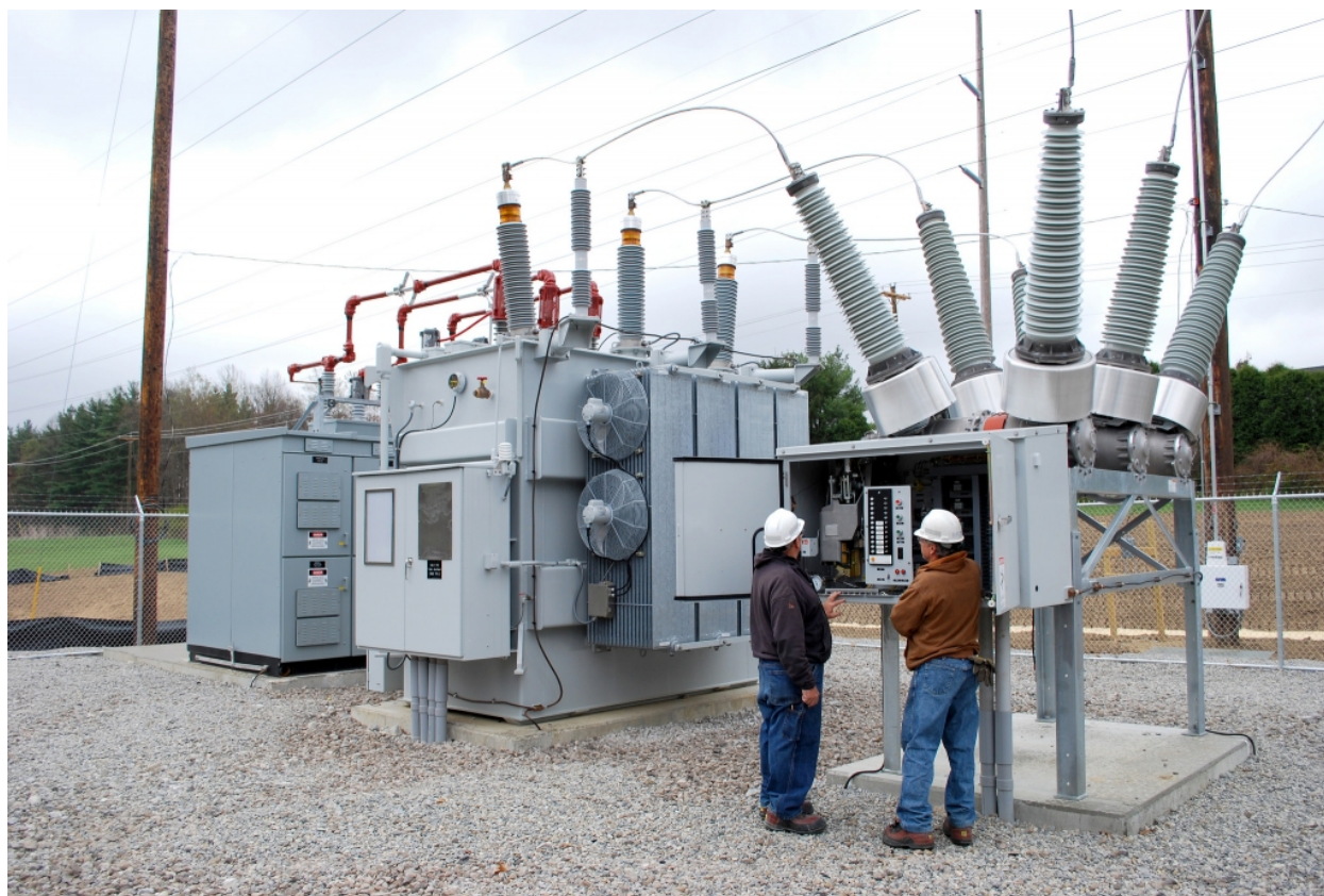
Figure 20: Substation Power Transformer. Three-phase substation power transformer steps down electricity voltage for local distribution system. Note the connected circuit breaker with swinging control housing doors near transformer. The control circuits for both transformers and circuit breakers are likely to be vulnerable to the E1 pulse from HEMP. Photo credit: First Energy.
