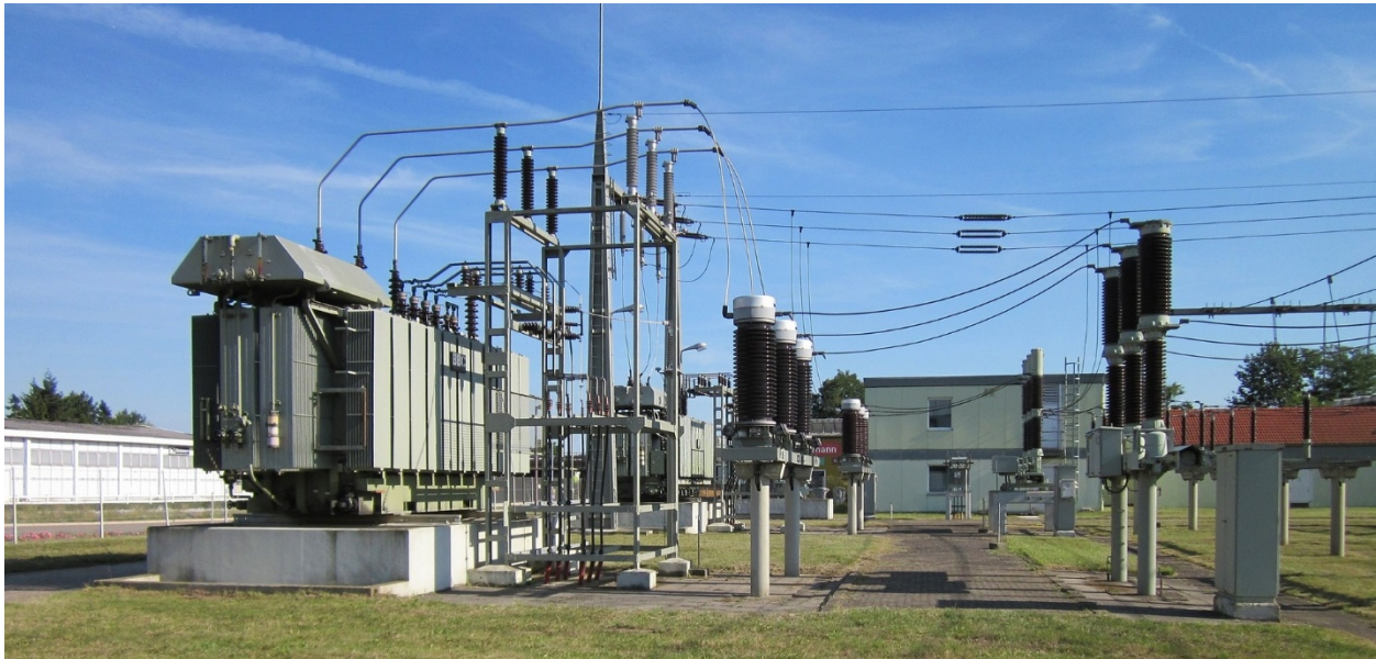
Figure 26: Instrument Transformers in Substation. Instrument transformers sense voltage and current by means of the transmission line conductor passing through an annular core wrapped with copper windings. All three phases of current pass through this inline set of instrument transformers to the right of the power transformers. Photo Credit: Pixabay .
