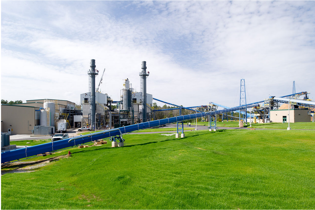
Figure 11: Biomass Generation Plant. The 20 MW Savannah River Site Biomass Cogeneration Facility in South Carolina replaced a coal-fired plant. This plant burns forest residue. Note the complex fuel handling system in the foreground, which may be vulnerable to the E1 pulse. Photo credit: U.S. Department of Energy .
