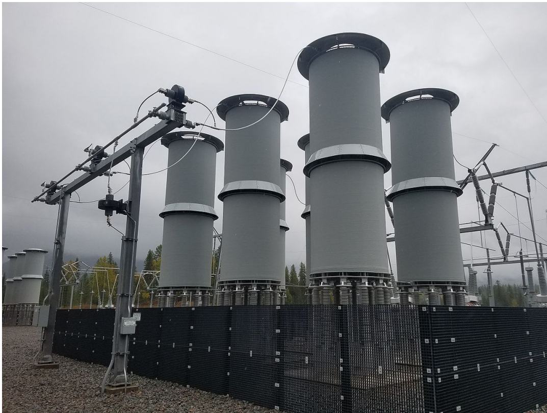
Figure 28: Substation Shunt Reactor Air core shunt reactors at a substation in Montana near the Noxon Rapids hydroelectric generation dam are designed to absorb reactive power. The spinning generators at hydroelectric plants produce large amounts of reactive power; shunt reactors balance this power during grid restoration. While shunt reactors operating at high voltage may be resilient to the E1 pulse, the vulnerability of their control systems needs engineering study. Photo Credit: Creative Commons/VARsity
