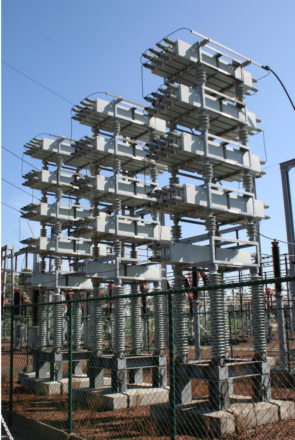
Figure 27: Substation Capacitor Bank Capacitor banks are installed in substations to provide reactive power support. Substation capacitors operate at the voltage level of the connected transmission line and, therefore, are expected to be resistant to the high voltage of the E1 pulse. Photo Credit: Wikimedia/Phillipe Mertens
