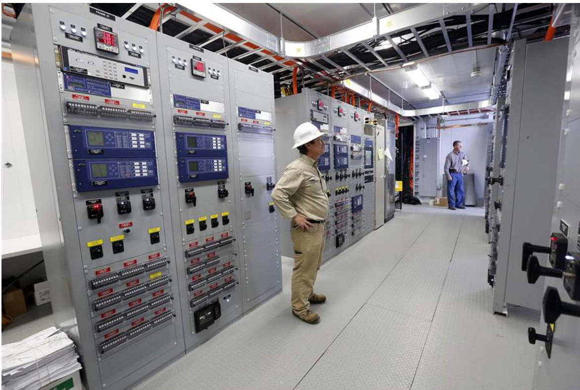
Figure 31: Rack Populated with Relays and SCADA in Substation Control House. SCADA, relays, and other digital equipment are typically contained in substation control houses. The E1 pulse, conducted into equipment interfaces, can cause upset and permanent damage. Photo credit: The Toronto Blade
