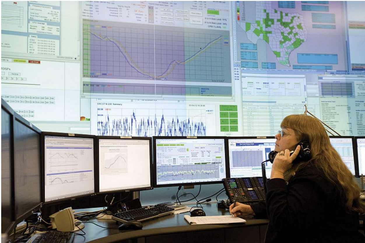
Figure 36: Reliability Coordinator Control Room. This reliability coordinator control room contains numerous monitors and large screen displays. The digital circuitry necessary to operate this equipment can be vulnerable to the E1 pulse. E3/GMD can cause harmonic effects misoperation of UPS if the control facility is unprotected. Photo Credit: Wikimedia Commons/Dpysh w.
