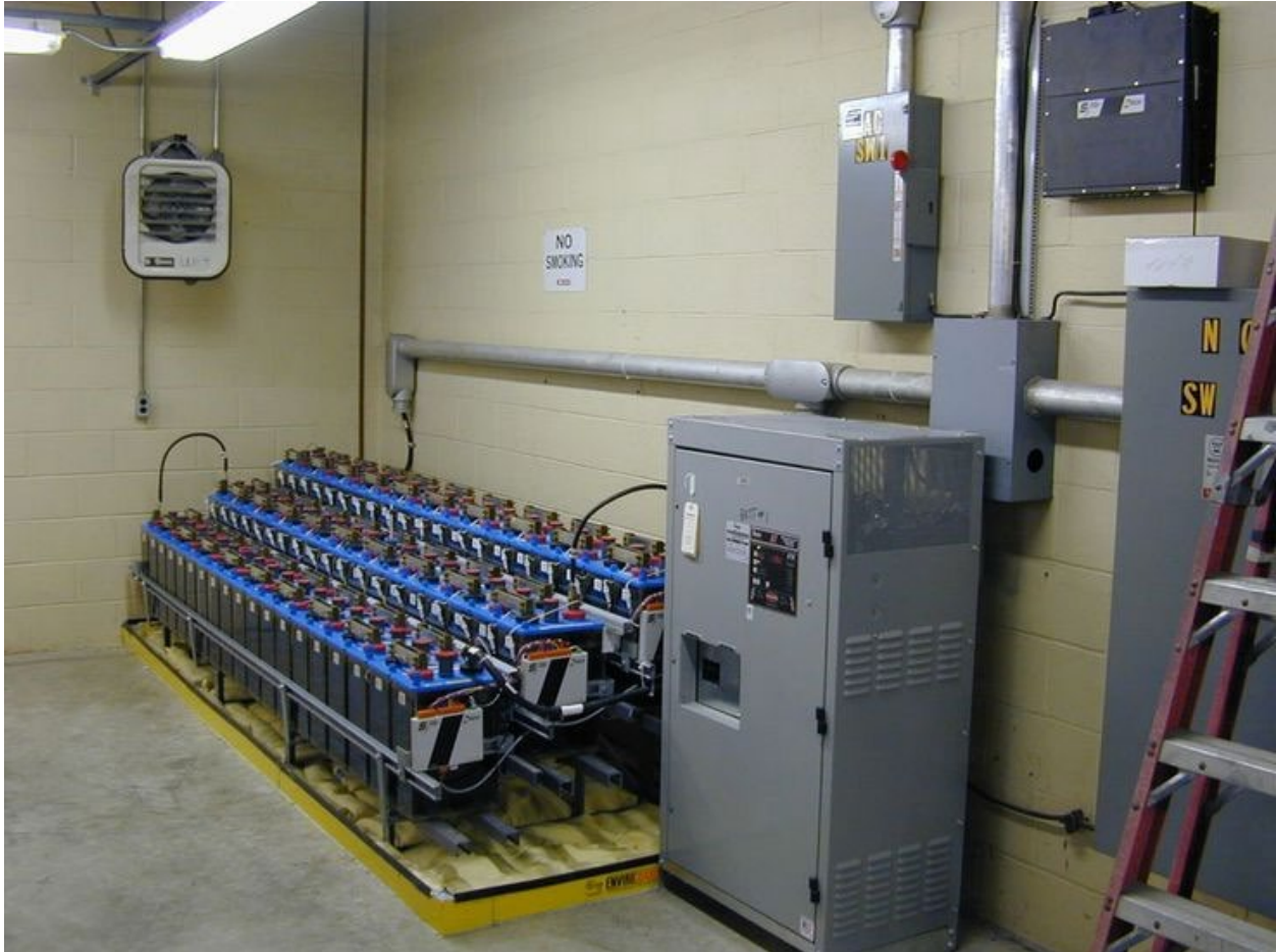
Figure 34: Uninterruptible Power Supply and Battery System. UPS and backup battery systems supply power to low-voltage substation devices, including circuit breakers, relays, and other control devices. Power leads into the UPS will conduct the E1 pulse and harmonics resulting from E3/GMD; malfunction or equipment damage could result. Photo Credit: BTECH
