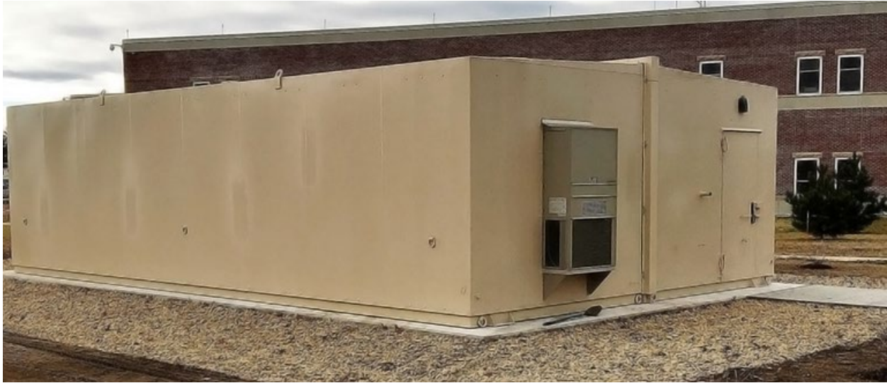
Figure 38: Shielded Control Enclosure. This modular shielded enclosure can be used at grid substations to protect relays, SCADA, and communications equipment. Photo credit: ARMAG Corporation
