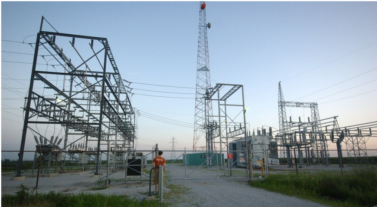
Figure 19: Bulk Power System Substation. Substations for the bulk power system transform high voltage electricity into lower voltages for homes and businesses. Circuit breakers at the left section of substation control power flow into high voltage transformers at the right. Communications for the substation are carried by microwave radio dishes on the tower at the rear. Open-air designs such as this expose substation components to the E1 pulse from HEMP. Photo credit: Creative Commons/ vaxomatic
