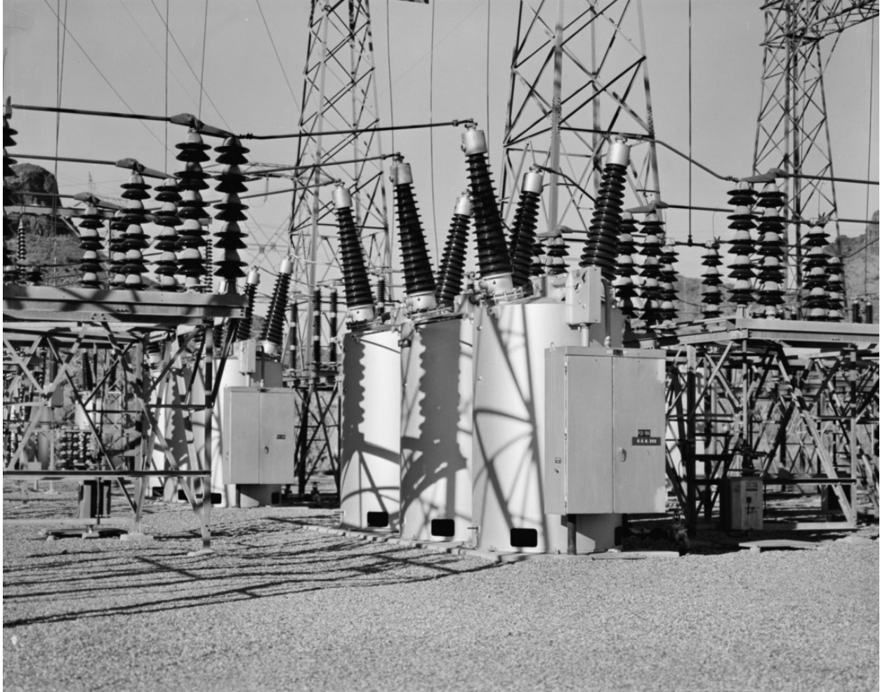
Figure 14: Generator Step-Up Transformers at Arizona-Nevada Switchyard for Hoover Dam. Single-phase generator step-up transformers raise voltage for long-distance transmission. During HEMP and GMD events, the transmission lines from Los Angeles to the switchyard can conduct geomagnetically induced currents into the windings of the transformers, causing overheating and harmonics. Without use of neutral ground blocking devices, harmonics can also be conducted into the dam's massive generators, causing vibrations and heating. Photo credit. Wikimedia Commons/Deborah Dobson-Brown .
