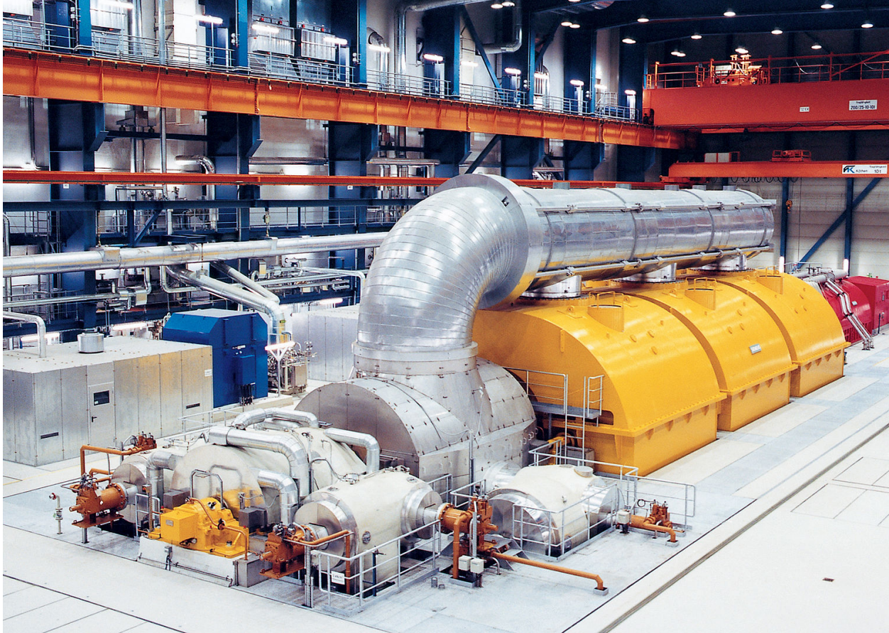
Figure 15: Generator Driven by Steam Turbine. Steam turbine (foreground) drives the electric generator (background). Generators can be vulnerable to overheating and vibration from harmonics caused by the E3 pulse and GMD. Photo credit: Wikipedia/ Siemens Pressebild
